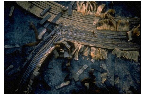
Melted 500kV transformer coil from EMP induced flux creating a hot spot
